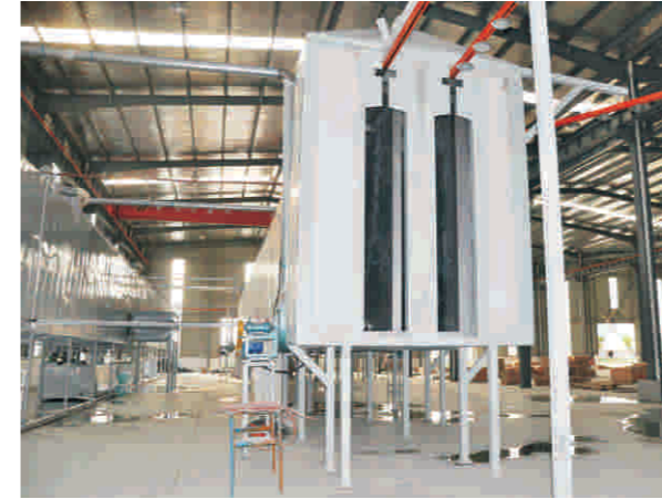
Tunnel curing oven and dry off oven
